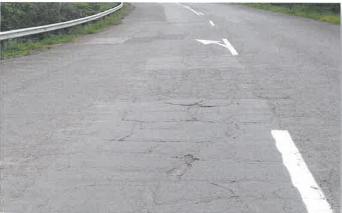
Severe block cracks at KM 21
