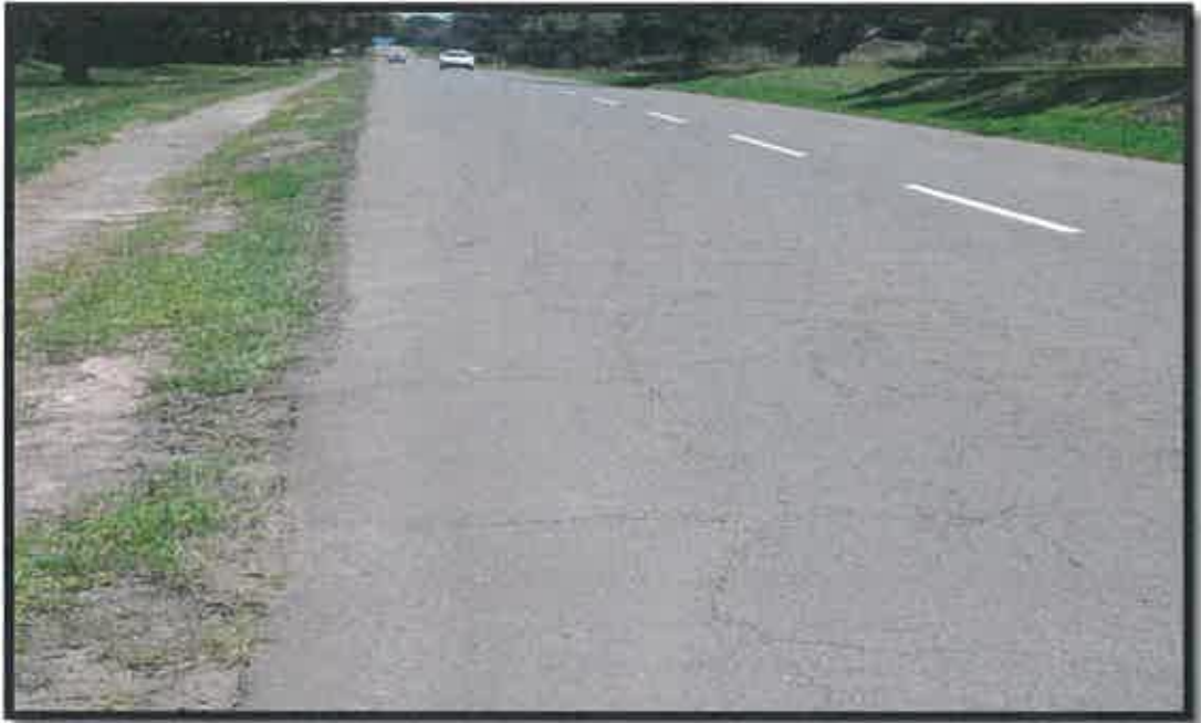
Figure 6: Block cracks at km 3.7
