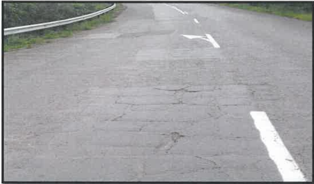
Figure 16: Severe block crack and surface crack at km 18.5
