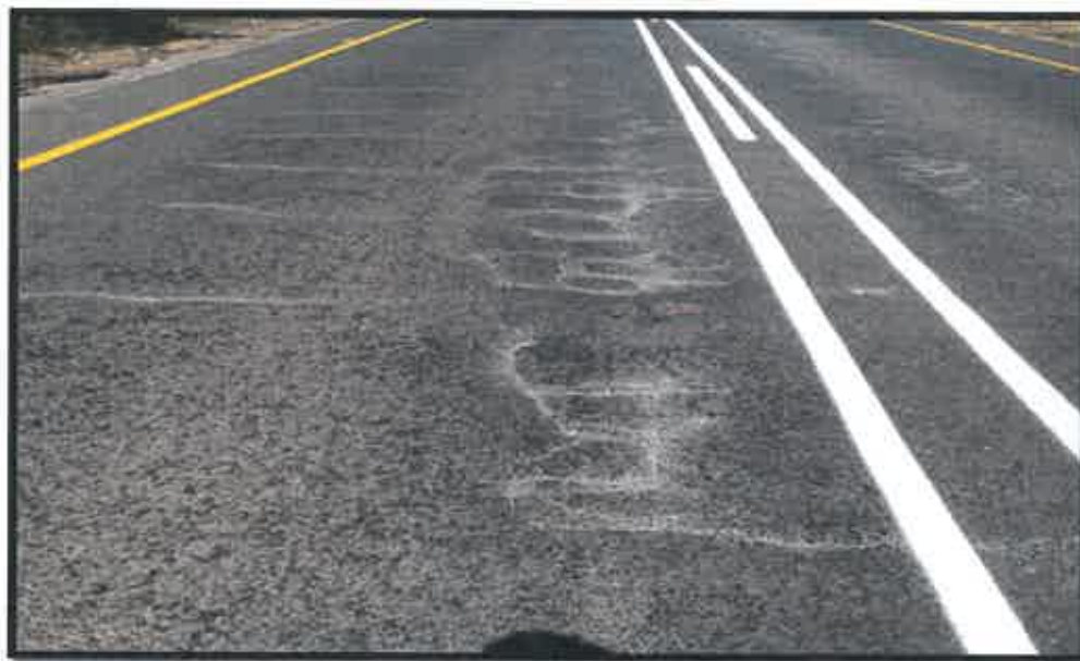
Figure 12: Block cracks with pumping at km 10.8
