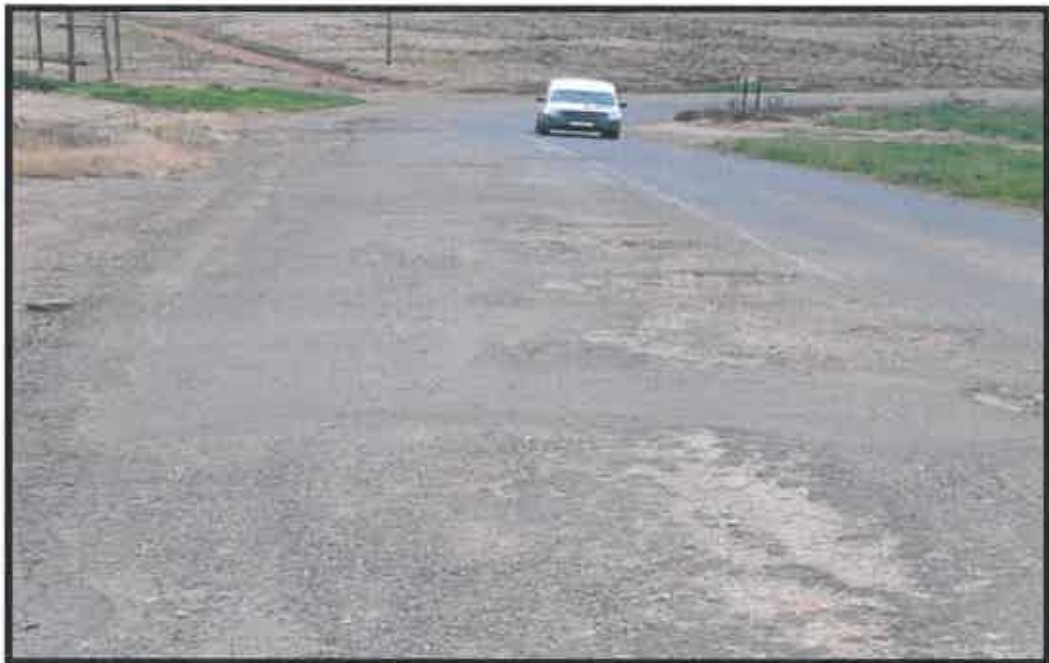
Figure 17: Extensive occurrence of potholes and patches at km 24.6
