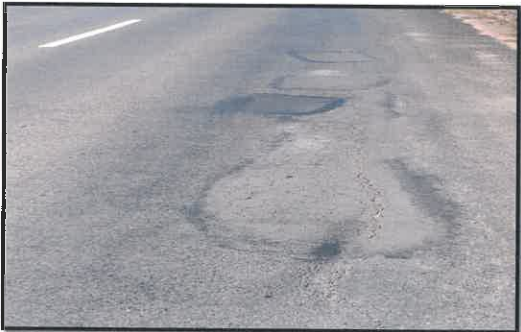
Figure 5: Multiple patches with cracks at km 3.4
