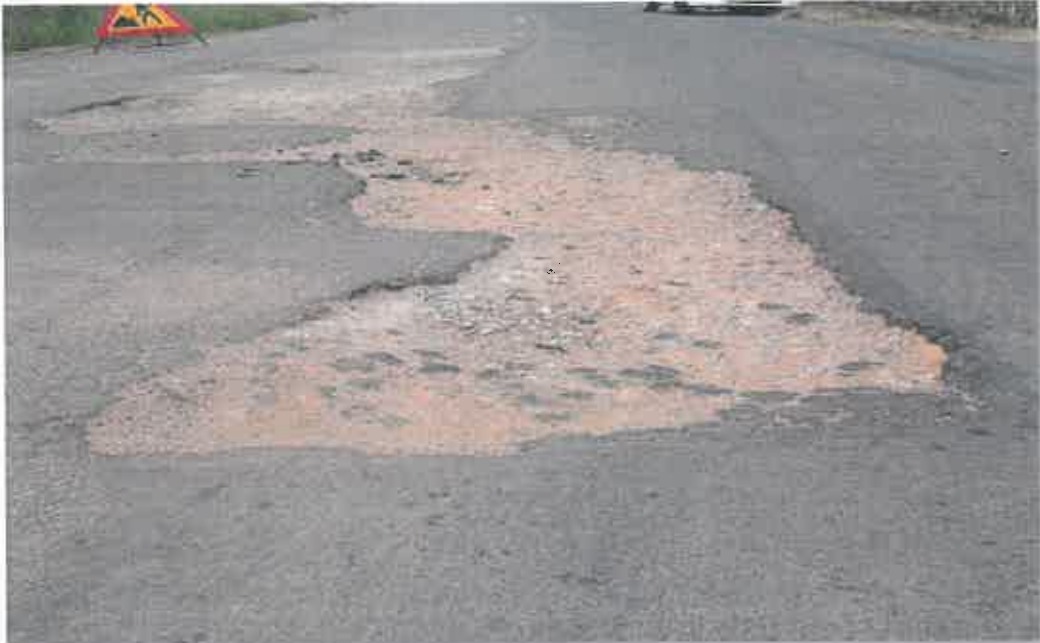
Structural failure and exposure of the base layer at Km 24
