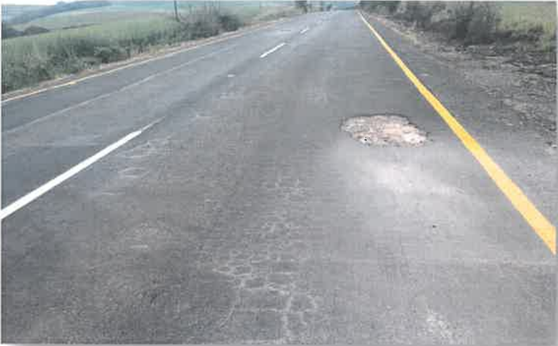
Crocodile cracks with pumping and pothole at Km 20.
