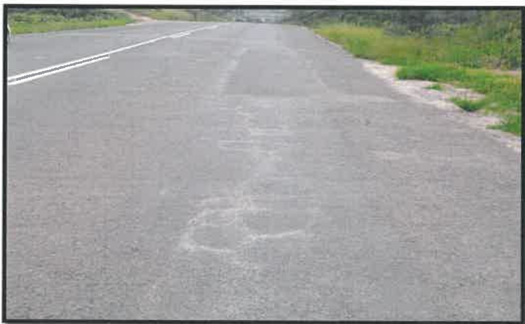
Figure 15: Block crack and asphalt patches at km 17.4
